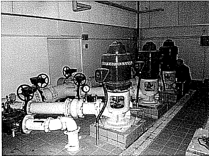
Photo 1 Service Pumps and pressure relief valve
